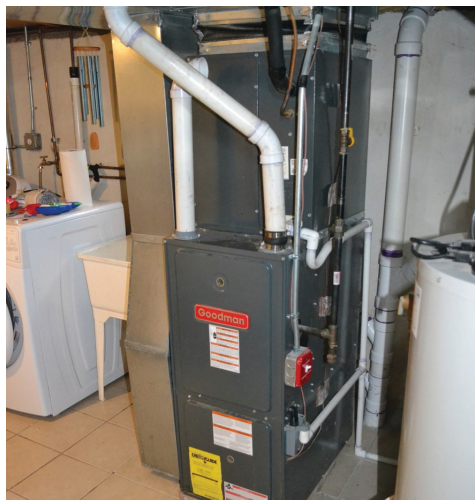
A typical forced-air furnace using gas heat and a cooling coil close-coupled to the top of the furnace
