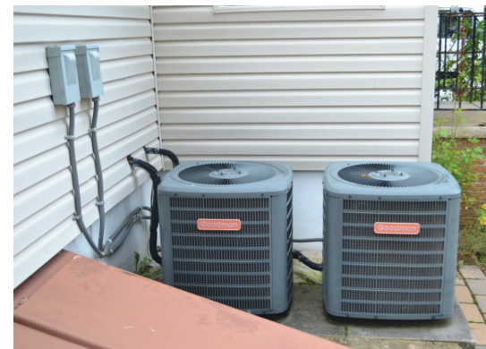
Two condensing units installed outside, but on a wall near the two furnaces in the basement
